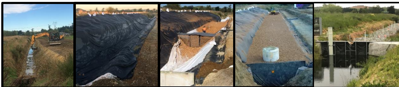
Figure 1: Photos showing various stages of the in-stream bioreactor construction. (left-right): drain clearance; laying of the EPDM rubber liner in which the bioreactor is sealed; filling the bioreactor with woodchip – concrete panel that acts as a dam end can be seen in foreground; bioreactor filled with 430 m 3 woodchip - ready to be sealed and plumbed (orange dot marks where inlet pipe was later fitted); completed bioreactor headworks – dammed drain water flows through the woodchip bioreactor under an ambient hydraulic gradient. Under storm flow conditions excess water spills over the top of the bioreactor. The white riser pipes protruding from the top of the bioreactor are monitoring wells that permit water sampling along the length of the bioreactor.
